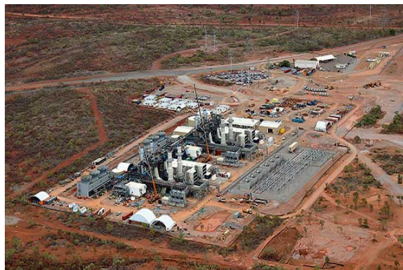
Diamantina Power Station, Mt Isa
